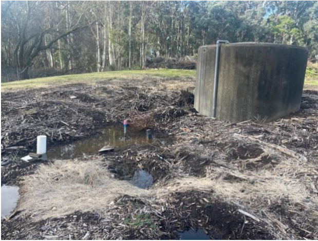
Water pooling near rainwater tank
