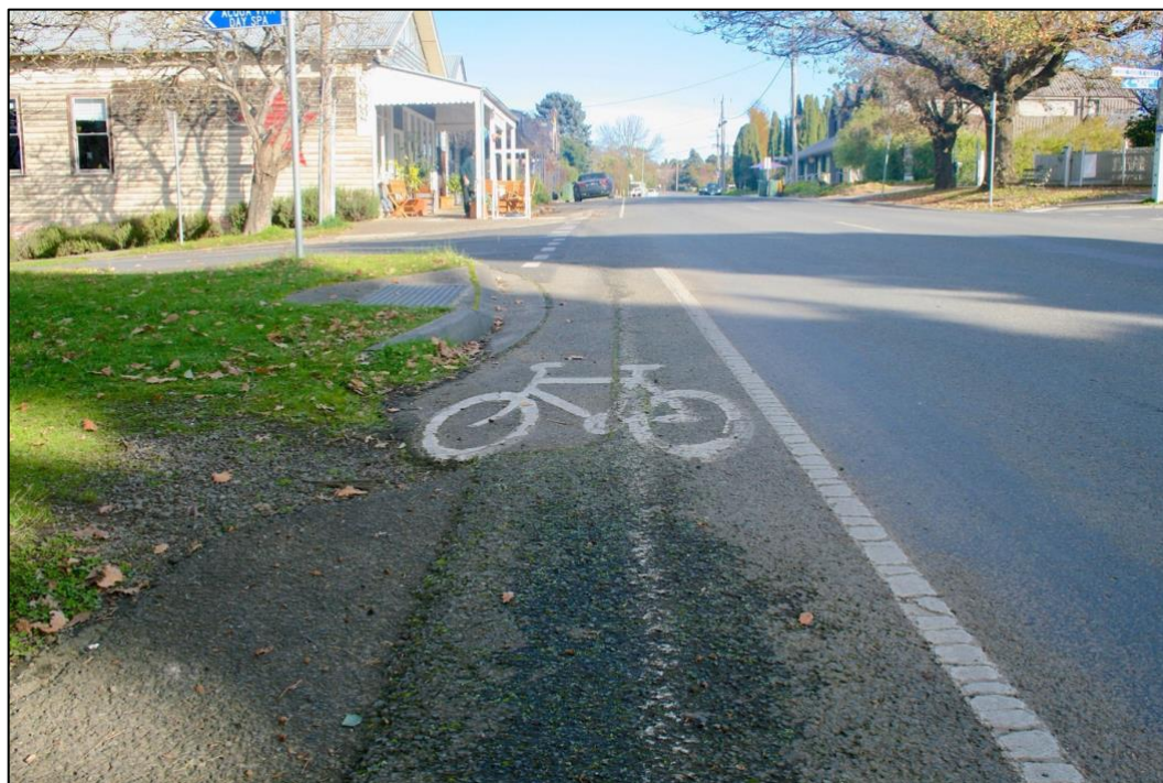
Figure 5.2: Narrow, uneven and incomplete bicycle lane in Hepburn Springs
