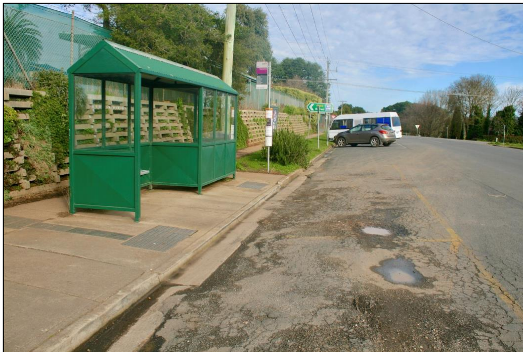
Figure 3.15: Damage to road surfacing, Bridport Street
