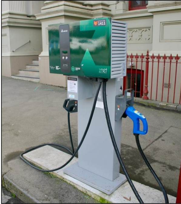
Figure 5.5: EV charging infrastructure on Vincent Street, Daylesford
