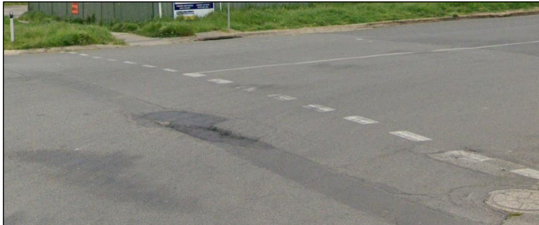
Figure 3.14: Road damage Bridport Street and Central Springs Road, Daylesford
